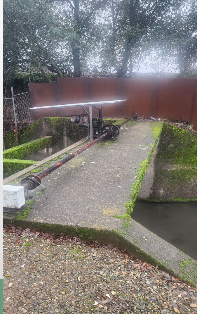
Main Canal Head gate
