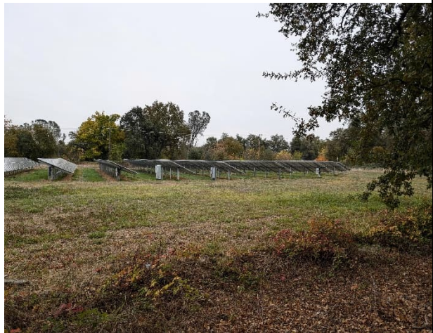
Figure 3-5. Photograph of Existing Solar Array Looking to the East
