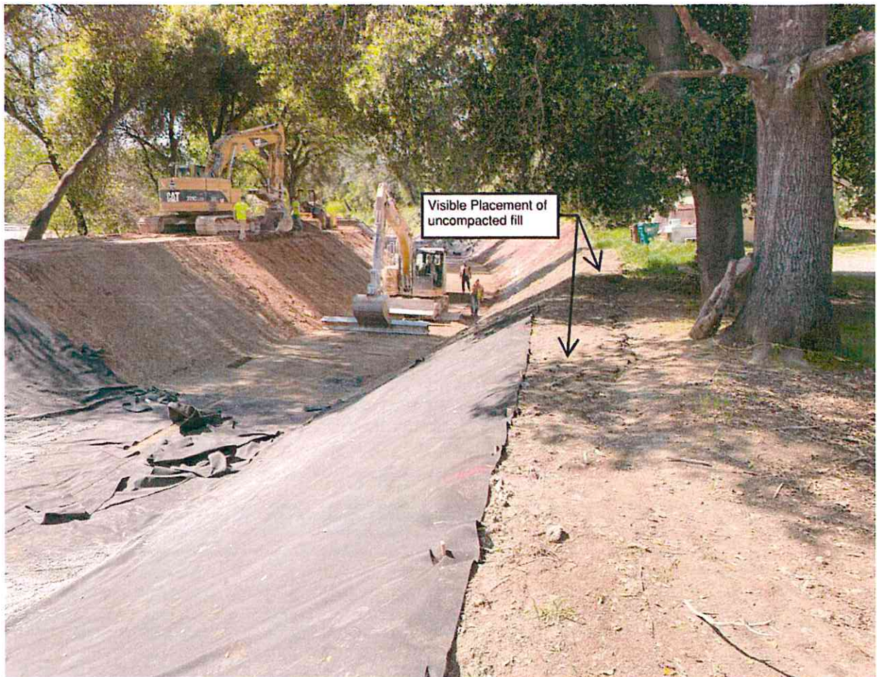
Image 3: Visible Uncompacted Fill
