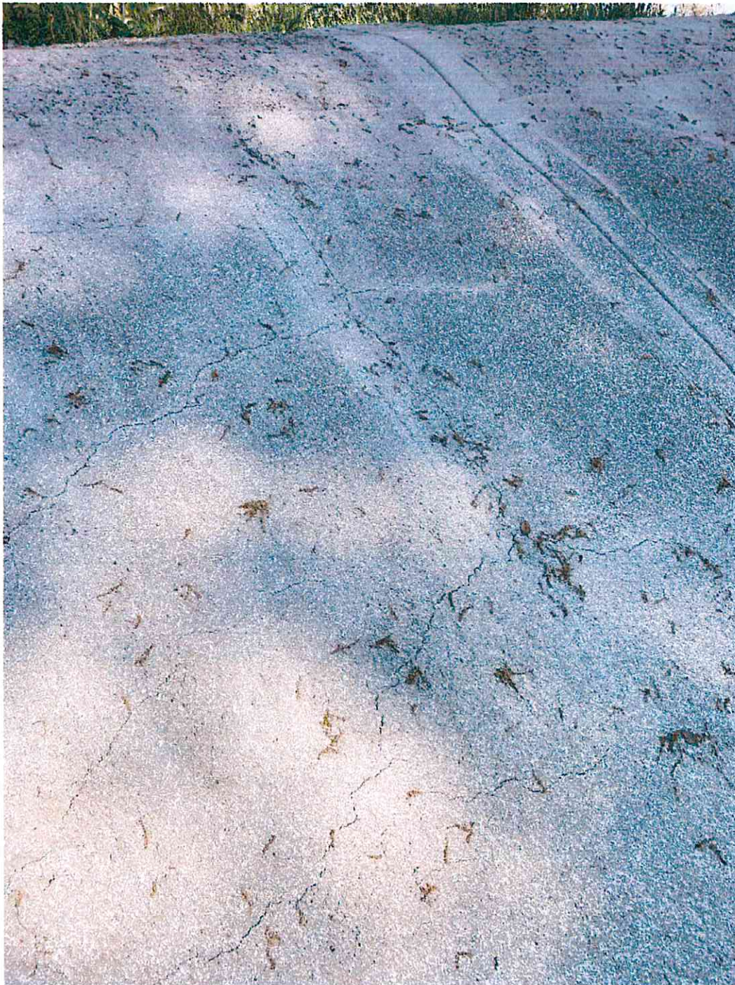
Image 1: Example of Observed Cracking of Recently Placed Shotcrete
