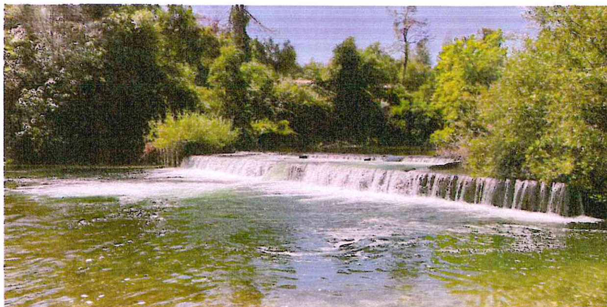
Figure 2.2 Existing conditions of sheet pile structure as viewed in August 2023 during NHC/CSS survey effort.
