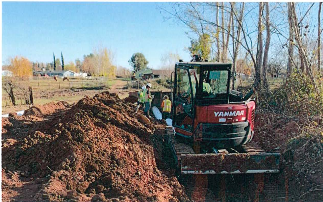
Pipe Installation ACID crew and rented mini excavator on Lateral 33 near Venzke Road
