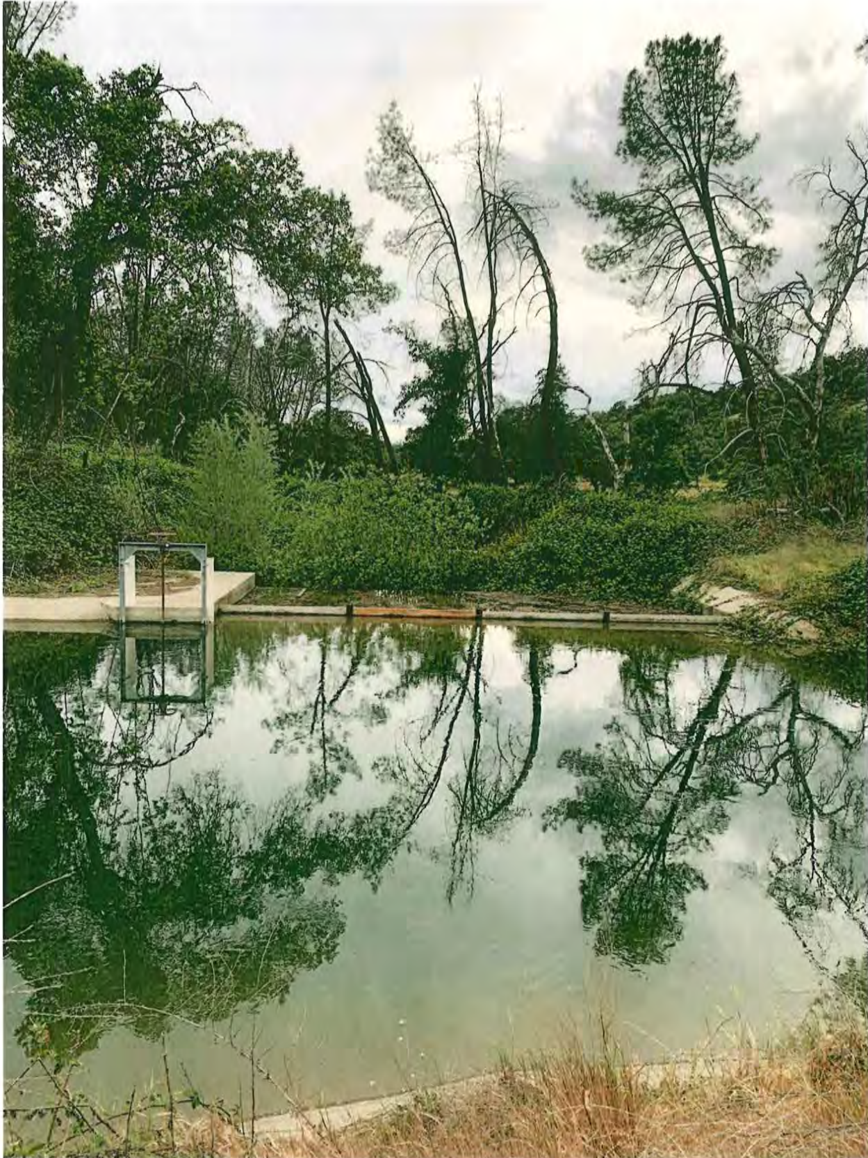
Canal height and spillway prior to vegetation removal and inspection on April 24, 2021
