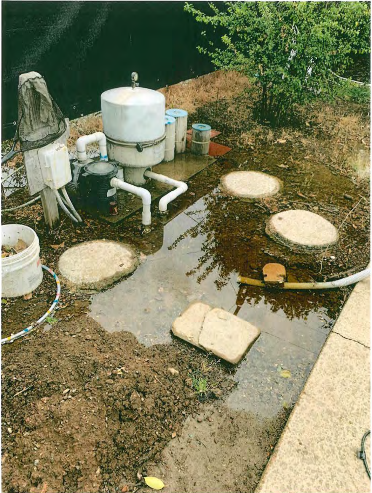
Lucille Yard Flooding First Reported on April 24, 2021
