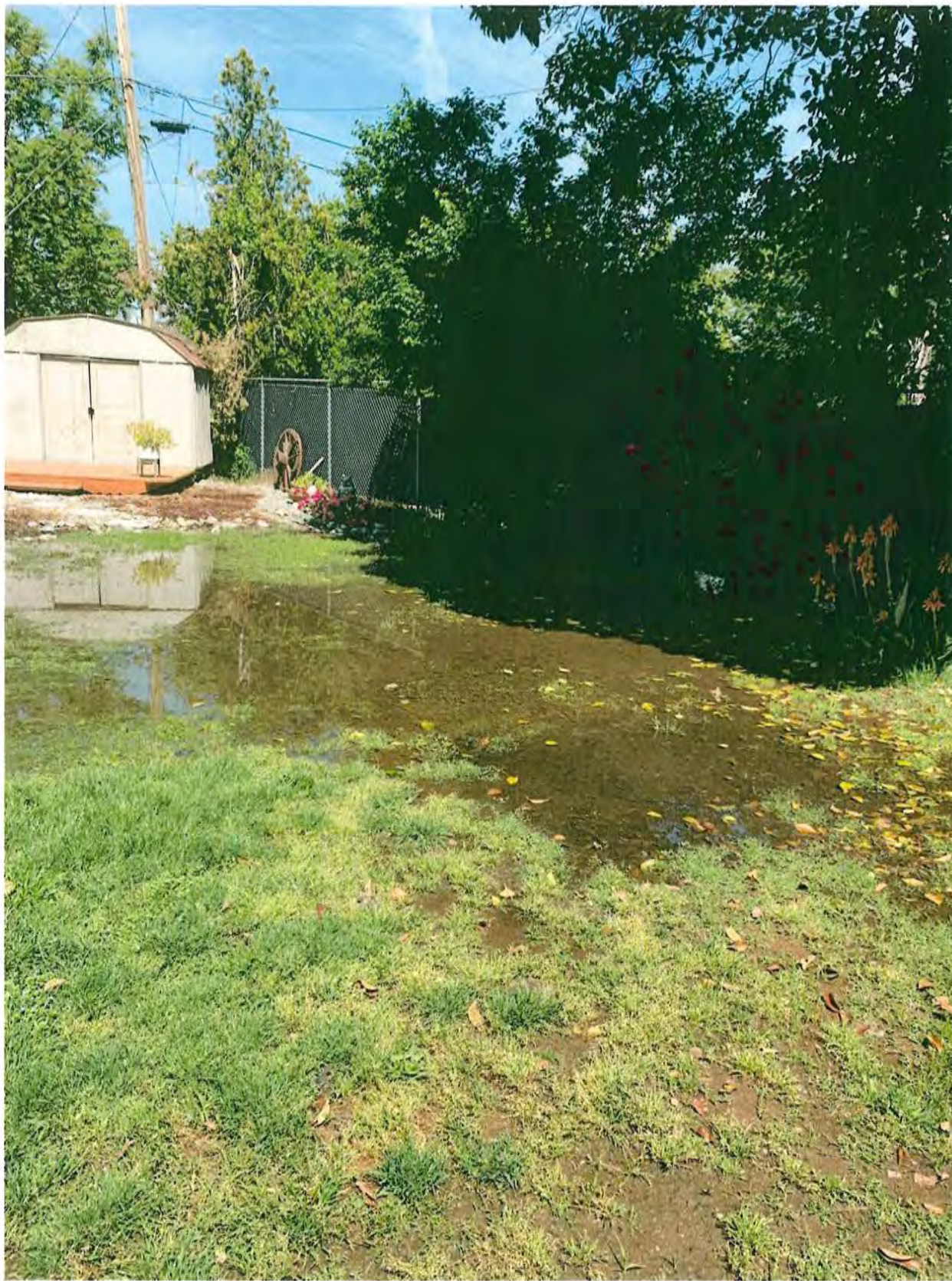
Yard Seepage on Lucille Street on April 29, 2021
