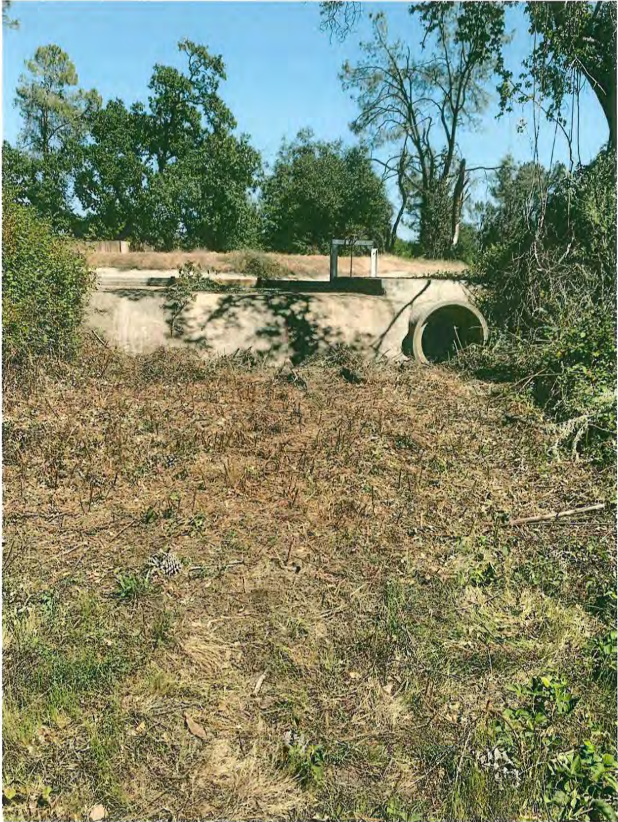
Area behind spillway after vegetation remove, inspection and water removal on May 2, 2021
